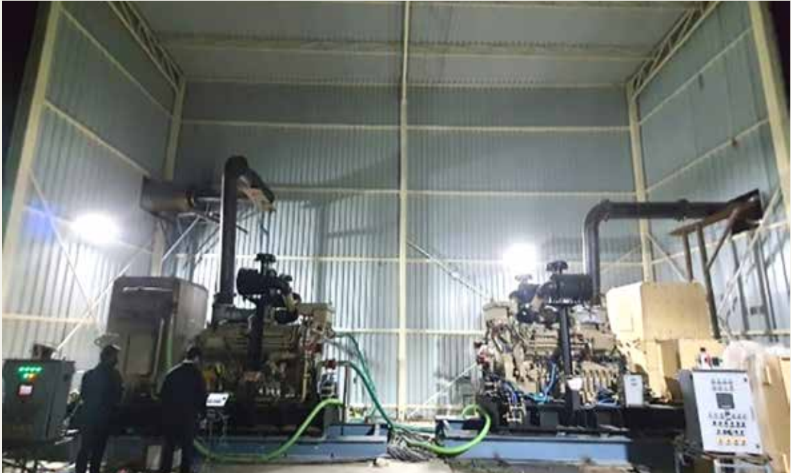
Marine Generator Set Testing Facility
